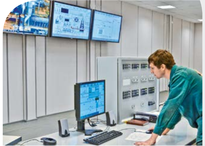
The modular BFXpert® automation system enhances the process control in blast furnace plants.
